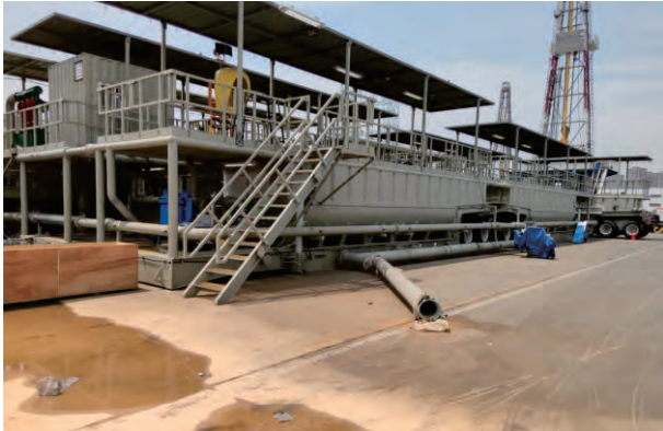
Trailer mounted tank
